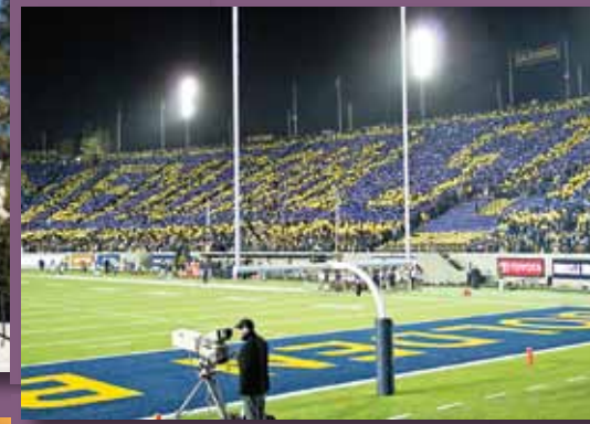
California Memorial Stadium opened its gates on September 1, 2012 after a 21-month renovation.
